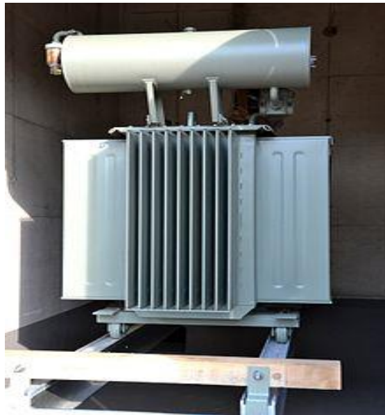
Figure 23. Oil transformer with air convection cooled heat exchangers
