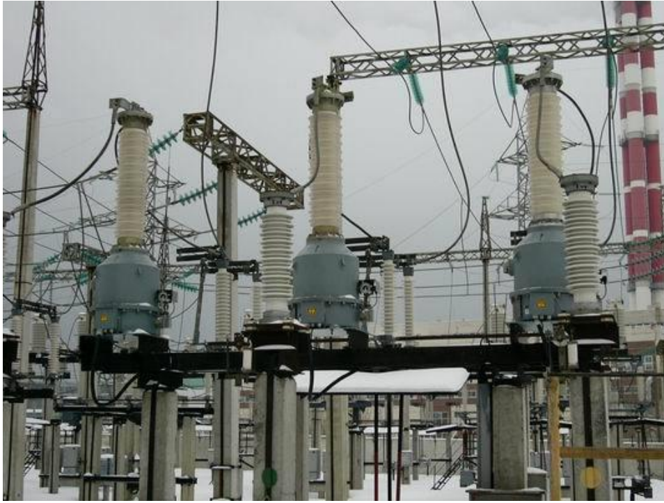
Figure 15. Potential or voltage transformer.
