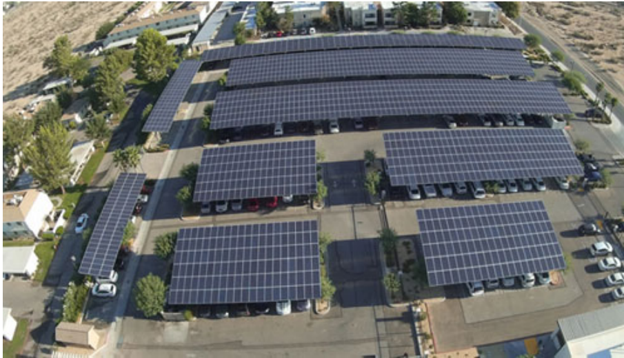
Obrázek 6.6: Projekt solar carport, Victorville, Kalifornie Zdroj: https://www.eastwest-bank.com/ReachFurther/News/Article/Ingenious-Hack-Solar-Parking-Lots-That-Generate-Power
