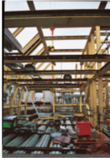
Figure 1.5 Slim-floor behind the retained façade (The free encyclopaedia for UK steel construction information, 2016)
