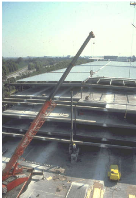
Figure 1.6 Dismantled and relocated steel car park, Munich (The free encyclopaedia for UK steel construction information, 2016)
