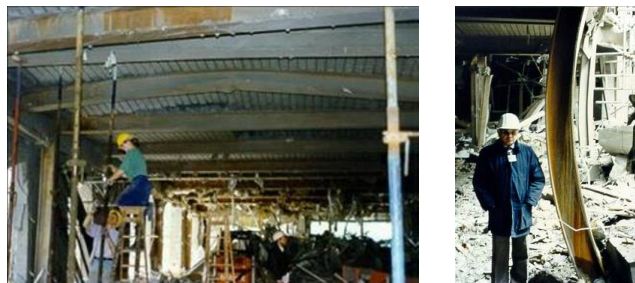
Figure 1. Exchequer Court bombing, St Mary's Axe, London 1992: a) damage to composite floors; b) ground floor steel columns [17]
