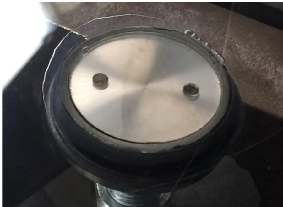
Figure 4.25 Glass-foil delamination (F1-03)
