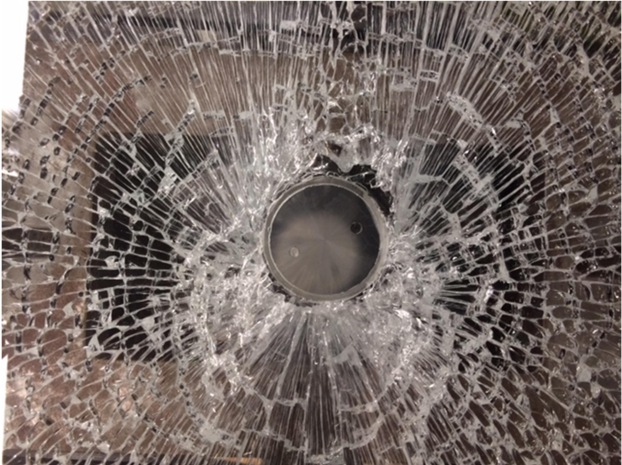
Figure 4.26 Destroyed heat-strengthened glass pane with the connection fitting imprint, float glass pane is intact (F1-03)
