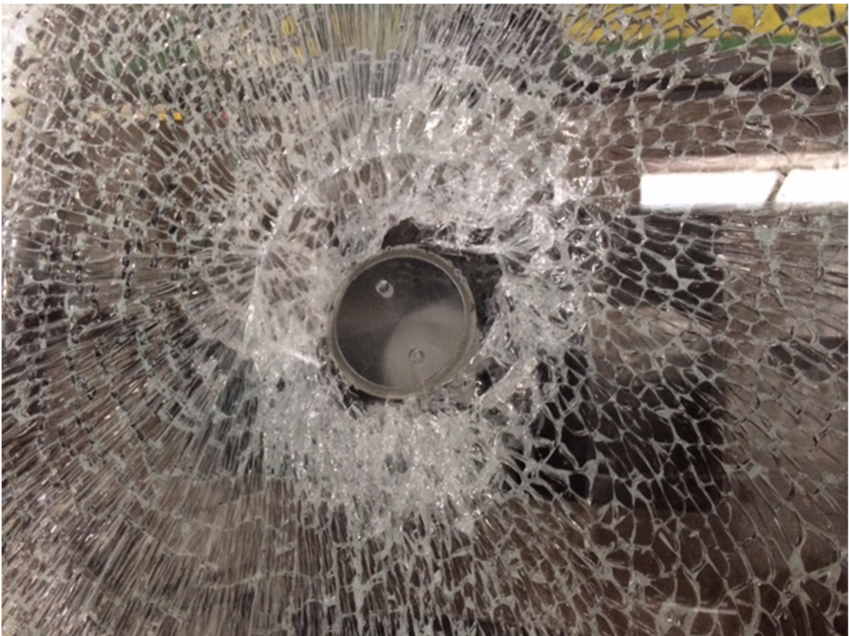
Figure 4.23 Destroyed heat-strengthened glass pane with the connection fitting imprint, float glass pane is intact (F1-02)
