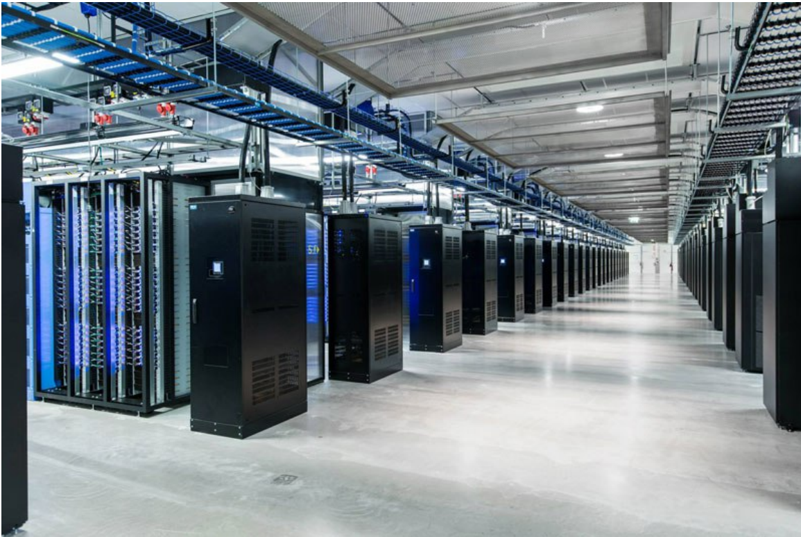
Figure 2.2: A data center interior example, Facebook, Inc., Sweden.
