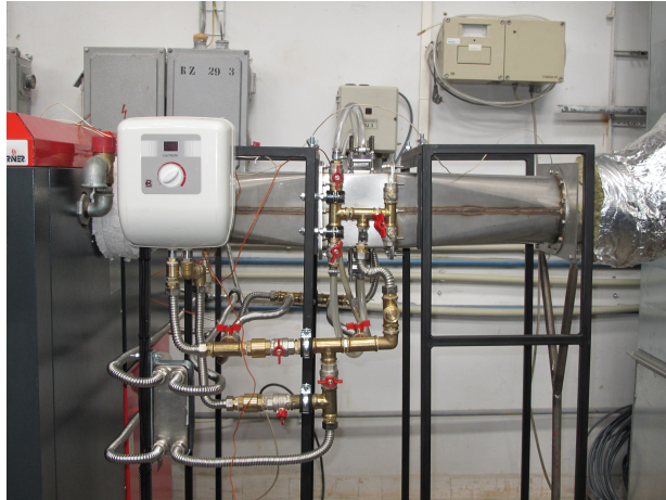
FIGURE 1. Thermoelectric biomass boiler test-system assembly.
