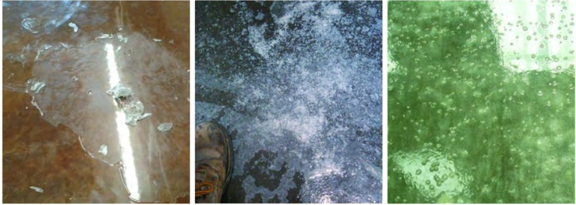
Fig. 3: From left to right: epoxy coating failure [7], blushing and bond failure, bubbles in a sealer [8]
