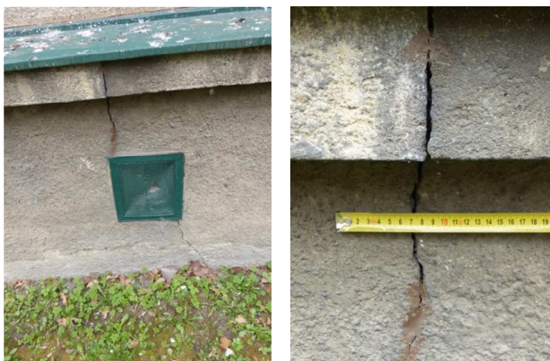
Obr. 2.6: Trhlina T02 - pohled a detail
