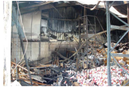
b) Collapsed warehouse
