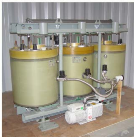
Completed transformer installed in container prior to connection
