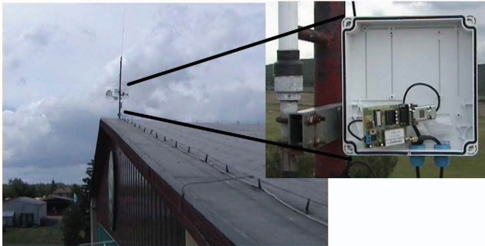
Figure 10. Receiver Antena and Receiver Module at LKMB Airport
