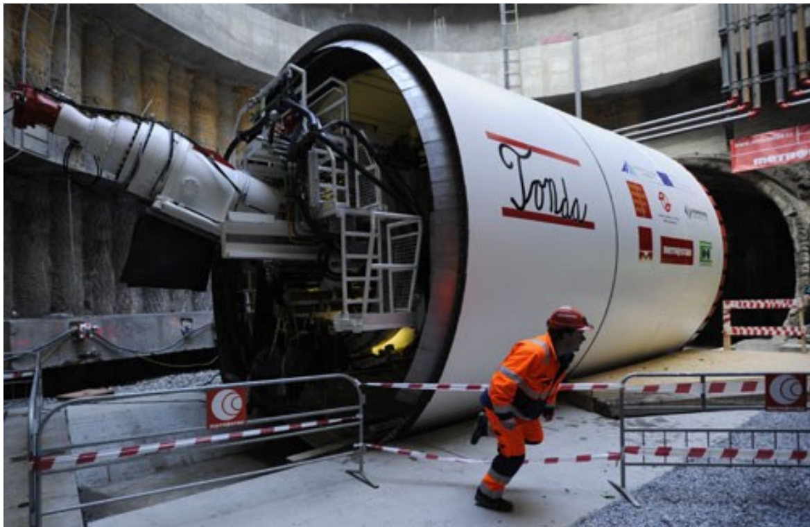
Figure 2.5: TBM used for excavation of underground line extension in Prague. Source: http://stavitel.ihned.cz/
