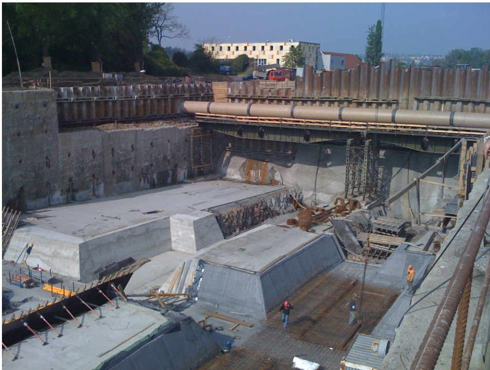
Figure 2.7: Blanka tunnel in Prague, Czech Republic, a section constructed with cut&cover method.
