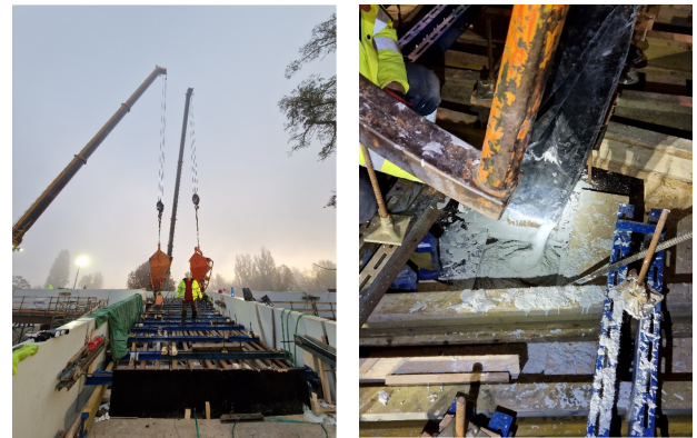
FIGURE 4. Casting process over the morning hours (left), filling hole during the casting (right).
