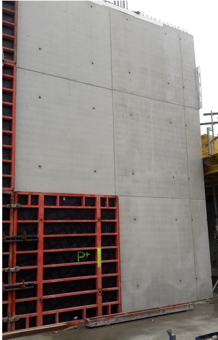
Figure 1.1: Example of a real-life faced concrete wall made out of self-compacting concrete on-site.
