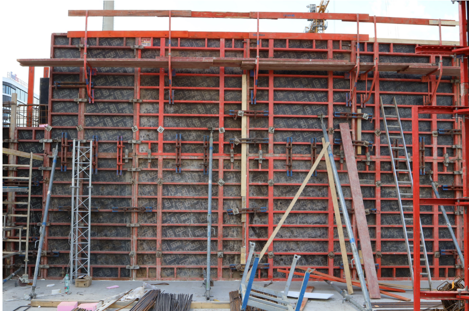
Figure 1.2: Example of a formwork of wall made out of self-compacting concrete on-site.
