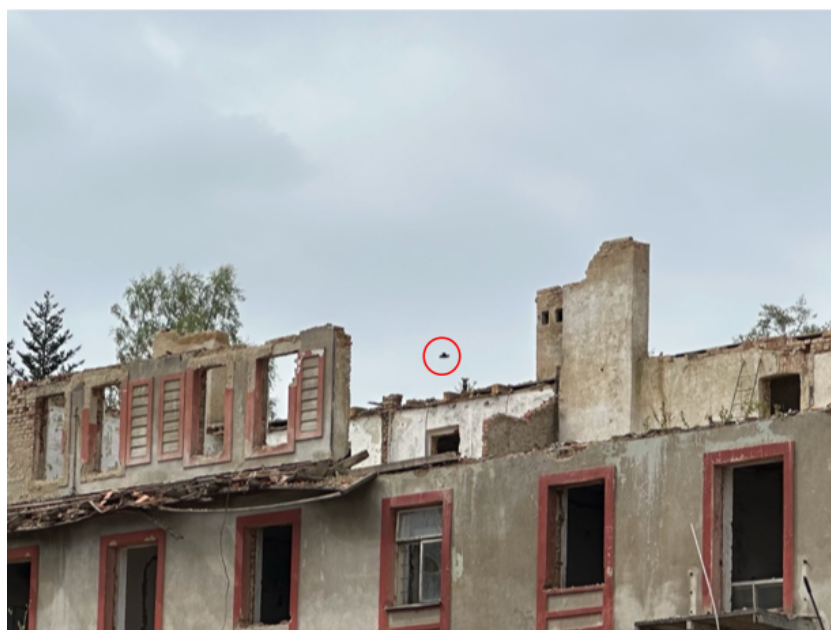
■ Figure 1.7 Use of FPV drone for detailed and rapid inspection (authors archive)
