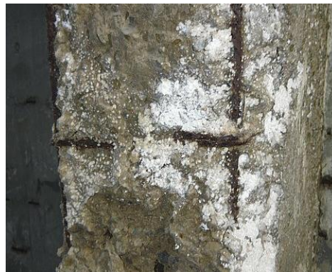
Figure 9: Type II corrosion (acid corrosion) Source: [F7]
