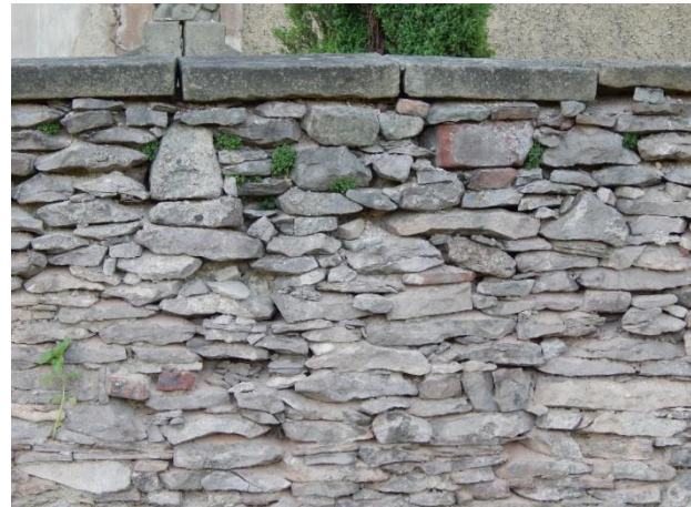
Figure 15: Biological deterioration Source: Author
