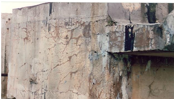
Figure 10: Corrosion III - sulphate corrosion Source: [F8]
