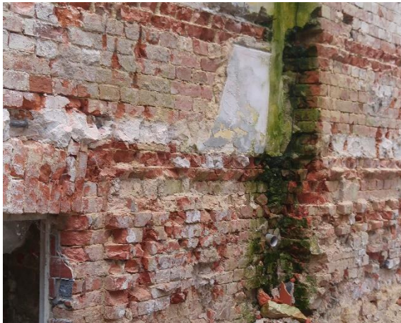
Figure 14: Biological deterioration Source: Author
