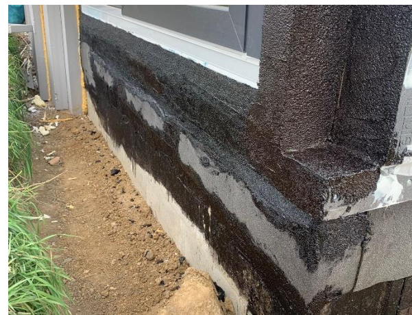
Figure 19: Application of the bitumen waterproofing screed on a detail with a complex shape Source: Author
