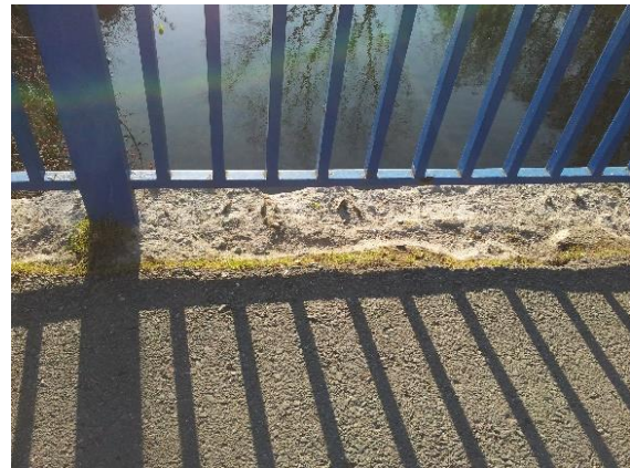
Figure 13: Bridge ledge deterioration Source: Author
