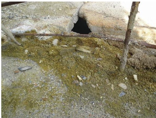
Figure 8: Type II corrosion (acid corrosion) Source: [F6]
