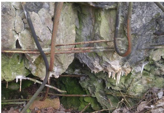
Figure 6: Corrosion I – leachates Source: Author
