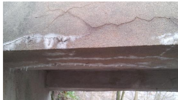
Figure 11: Corrosion III - sulphate corrosion Source: Author
