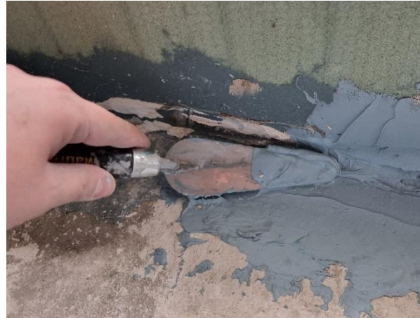
Figure 23: Application of the polymer waterproofing screed on the detail under the door
