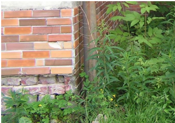
Figure 12: Surface damage Source: Author
