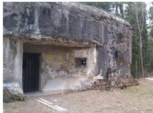
Figure 7: Corrosion I – leachates Source: Author
