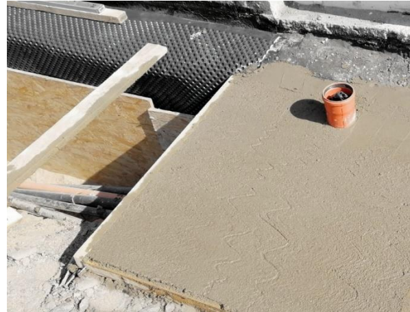
Figure 21: Application of the silicate (mineral) waterproofing screed on the drain area Source: Author
