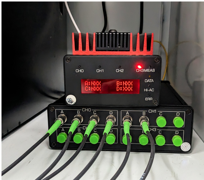
Figure 5.1: FBG interrogator unit placed on top of the switch.
