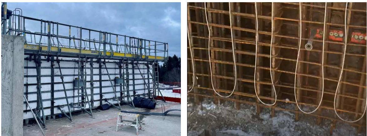
Figure 9 – Insulation of wall formwork (left), Heating of concrete with disposable cables (right) [Photo: R. Björkman, I. Beliatskli]
