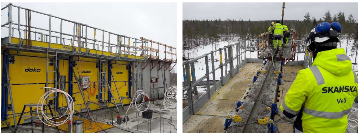
Figure 12 – Heated formwork in use (left), concrete pouring into the heated formwork in Finland (right) [Photo: author]
