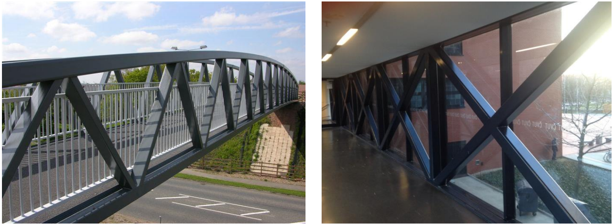
Figure 1.3 Examples of RHS application in bridges (left - Pedestrian bridge in Scotland (GB), right - Passage between buildings in CVUT (Czech Republic))
