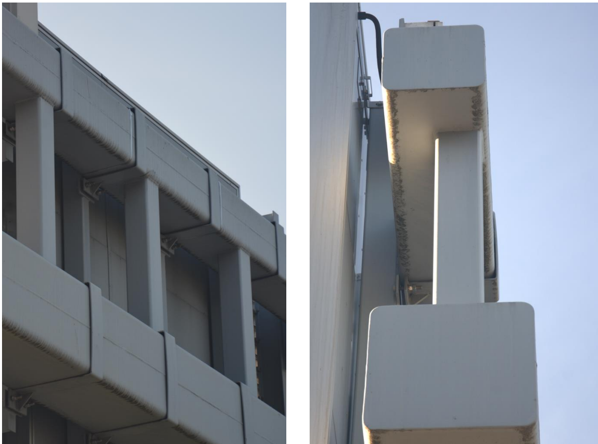
Figure 3.1 Stepped connection with eccentricity (SCE) in real-world design practice (photo: S. Kalmykova, Prague)
