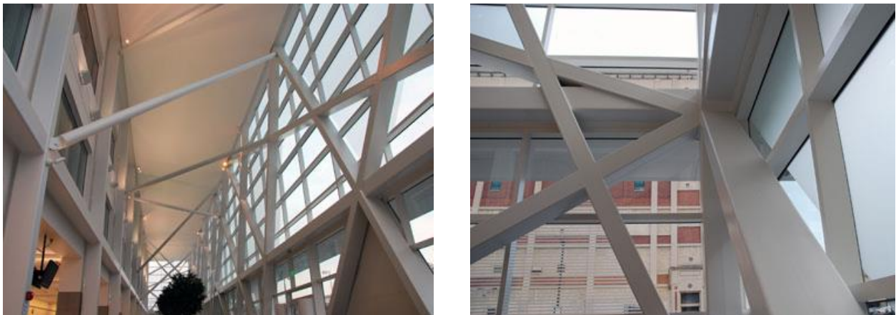
Figure 1.1 Examples of SHS application in bearing structures of transit terminals in Wisconsin (USA) and in Milwaukee (USA)
