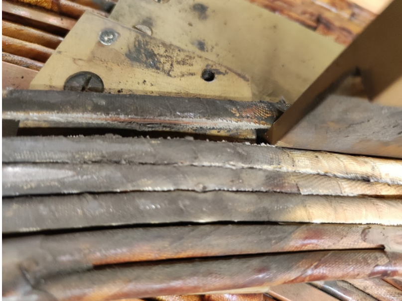
Figure 3.11: Detail of the trim coil No. 6 power leads breakdown.
