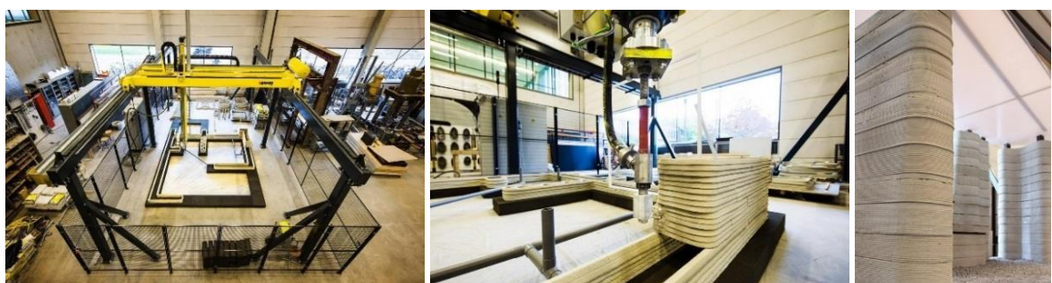
Fig.11: 3D printing at TUE, Netherlands a) Gantry 3D printer b) Printhead c) 3D printed wall detail
