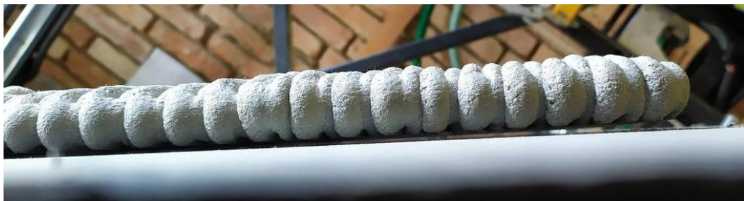
Fig.70. a) Panel end lifting due to different shrinkage 24 hours after printing
