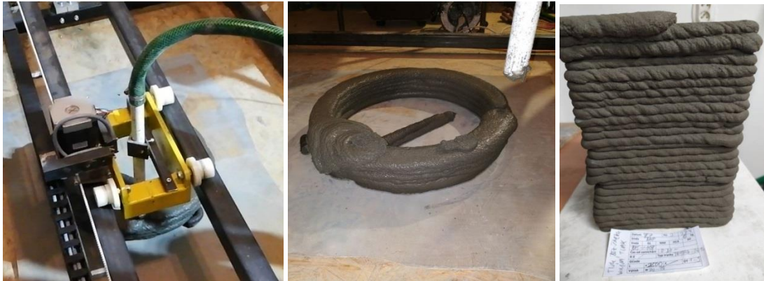
Fig.39. Printing by extrusion of DN20 pipe a) Set-up b) The first successful print of CM276 mixture c) Fluctuations in pressure and layer appearance when printing from a pipe without an auger and pressure control
