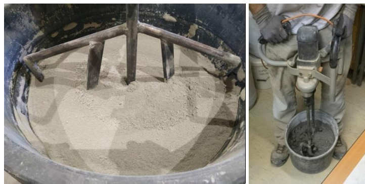
Fig.46. a) Mixing of dry components in custom-built mixing station b) Mixing of 018 kg of fresh mortar with MX 1600 DUO 2 gear stirrer with double whisks
