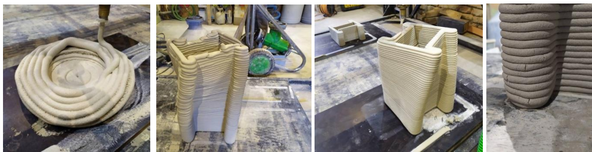
Fig.86. a) Sikacrete 751 3D printing test result No. 1 – Collapsed V-EGG-OUT object b) Sikacrete 751 3D printing test result No. 4, Sanax DT pump behind c) Sikacrete 751 3D printing test result No. 3 and No. 4 – top quality of H-O_050 objects d) Sikacrete 751 3D printing test result No. 4 - Detail of cracks within the bottom part of H-O_050
