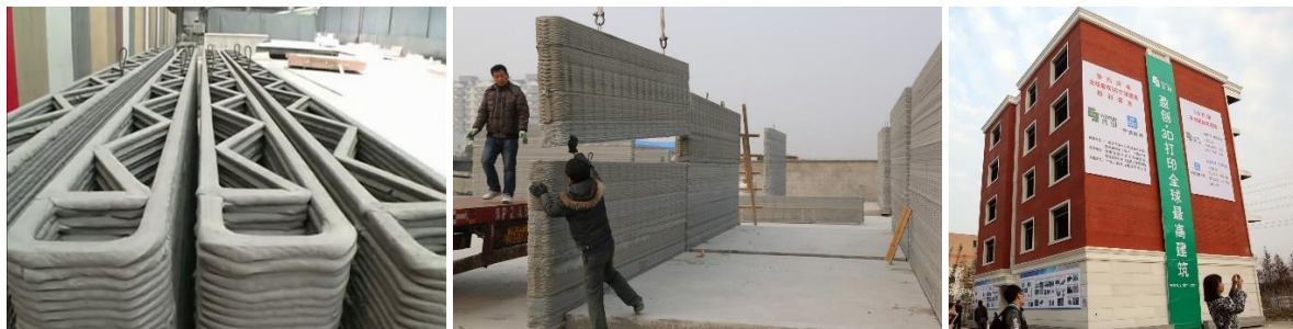
Fig.8 : 3D printing at WinSun, China a) 3D printed wall prefabricates b) Final assembly of walls c) 5 story residential building made of 3D printed wall prefabricates
