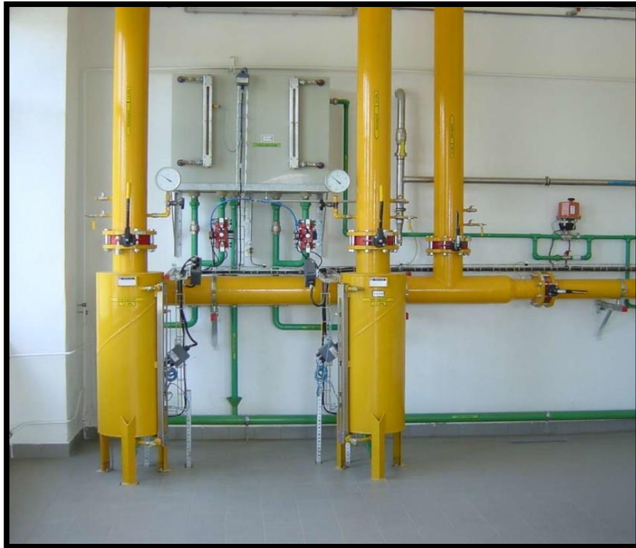
Figure 13. Heat exchangers for water vapor reduction [52].
