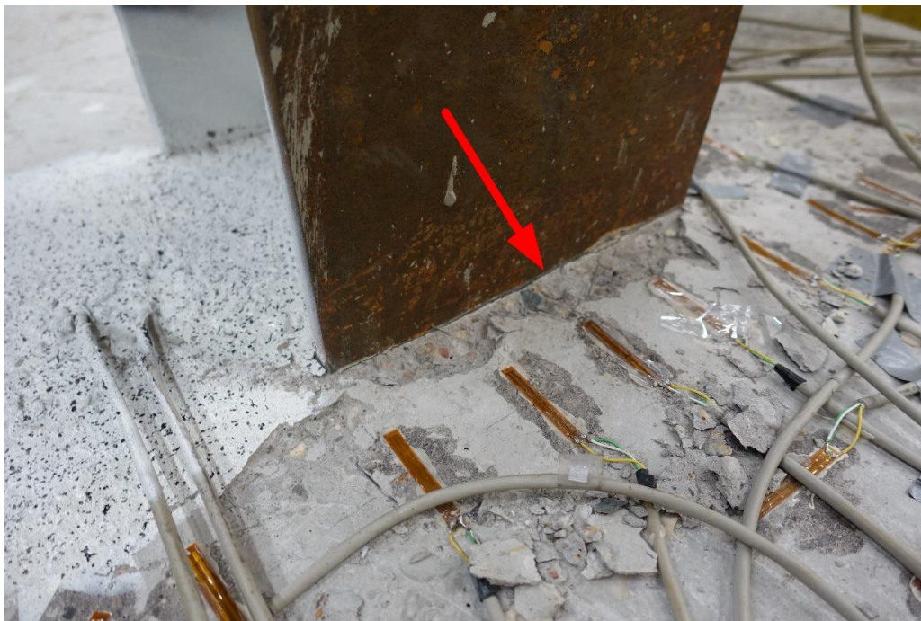
Fig. 53. Crushing the concrete slab in front of the column by a sagging bending moment.
