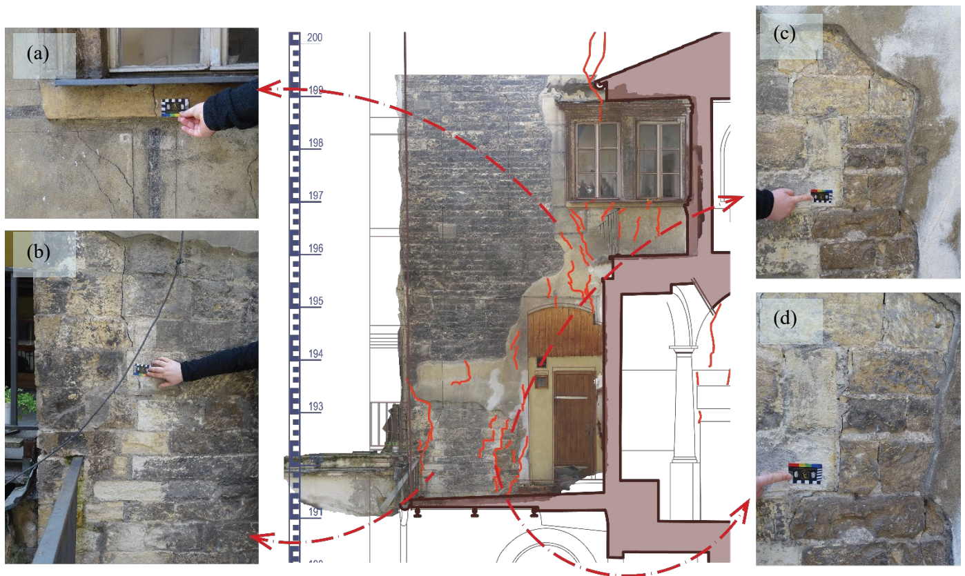
Figure 4.6 cracks mapping – Southeast corner of the Tower.
