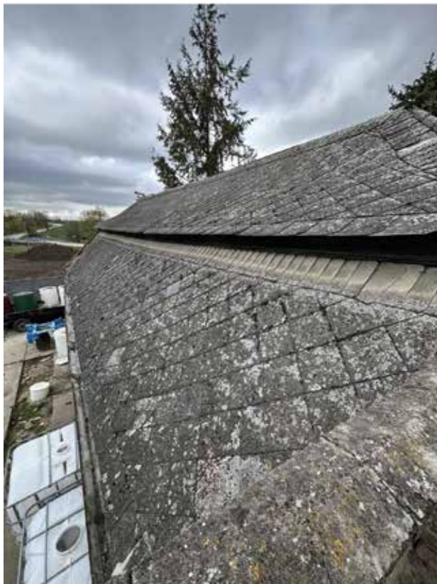
Fig 47: Degraded Eternit roof by biological colonization
