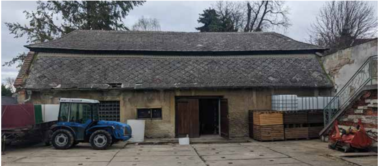
Fig 33: West facade is mainly covered by eternite roof with biological attack of lichee and moss.
