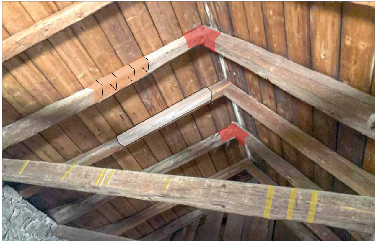
Fig 54: Truss type A North section with damage mapping
