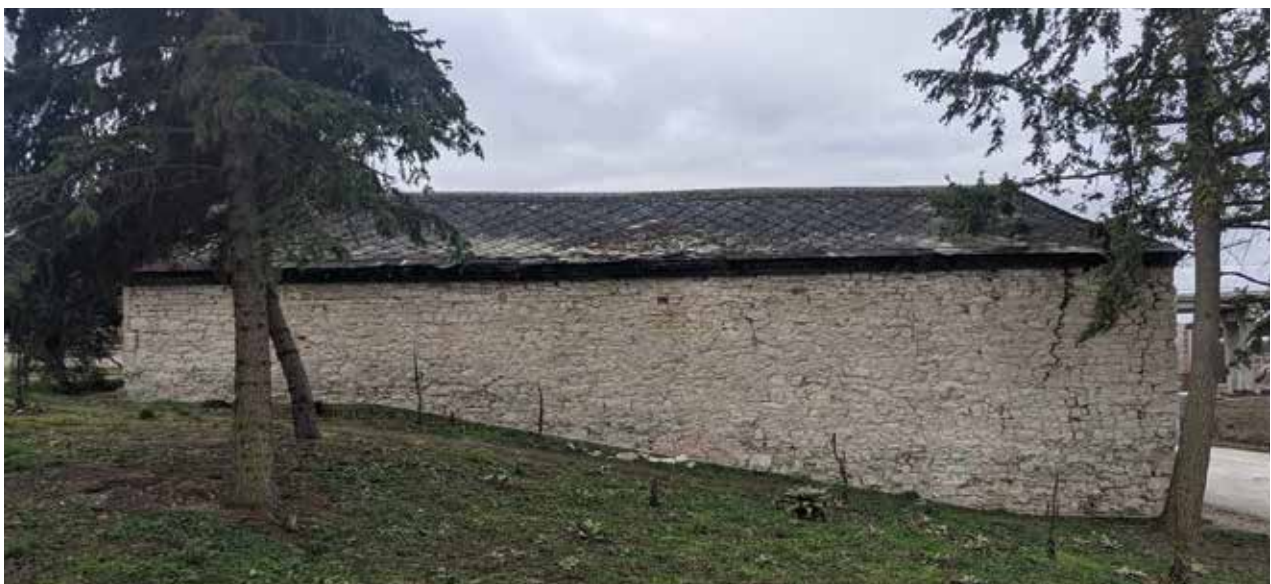
Fig 34: East masonry wall shows cracks in its colindance with the street and slope.
