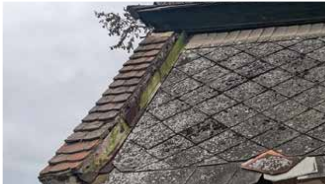
Fig 45: Moss growth in joints between masonry walls & eternite sheets
