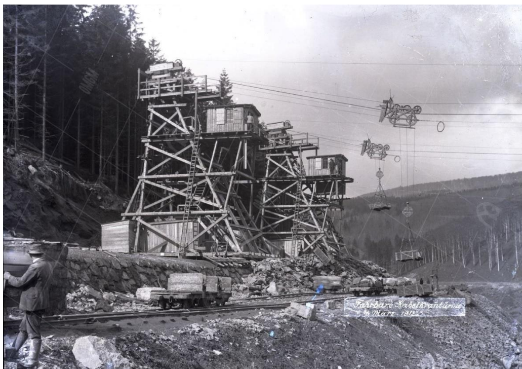
Figure 2.1 - Material transport in the Mostecká valley (a) picture of the wagons, August 20, 1911; (b) picture of the railroad, August 19, 1911; (c) picture of the cable crane tower, March 1912, © Panoráma starého Mostecka.
