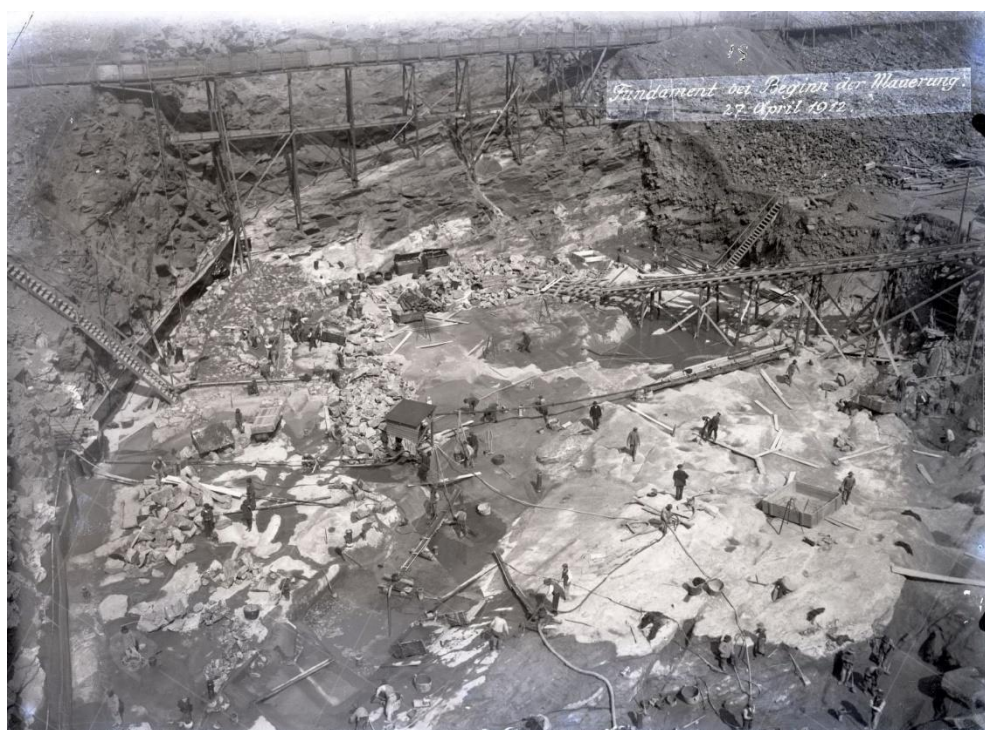
Figure 2.2 - Picture of the foundation joint of the dam, cleaned with pressurized water and steel brushes, 26 April 1912, © Panoráma starého Mostecka.
