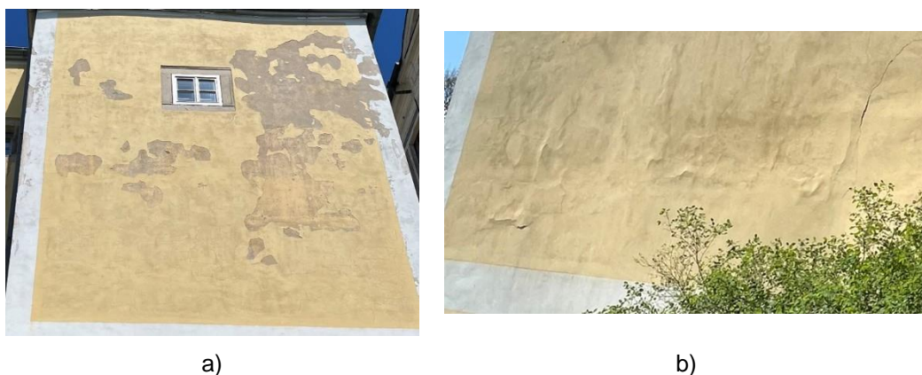
Figure 4.3 - a) Delamination of Southwest facade, b) Blistering of Southeast facade
