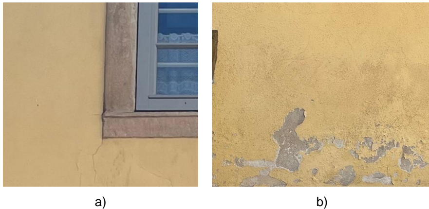
Figure 4.2 - a) Fracture crack near a window, b) craquelè effect
