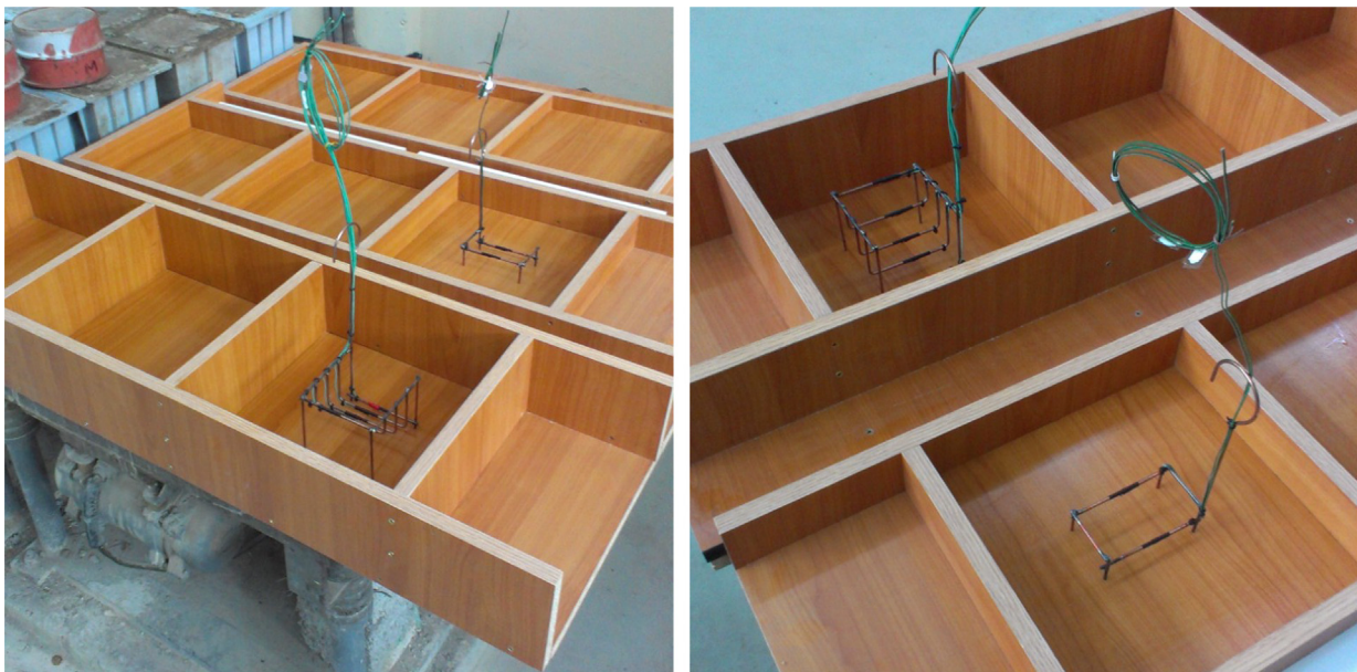
Fig. 1. Moulds for the wall-panel specimens and positioning and fixing of thermocouples, see also [24].
