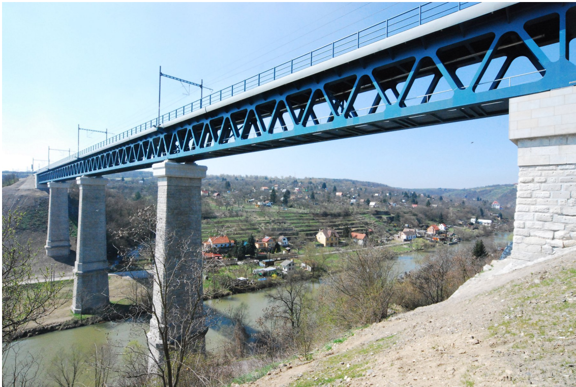
Figure 4.9: Bridge B5 – truss girder bridge with upper bridge deck and ballast bed.
