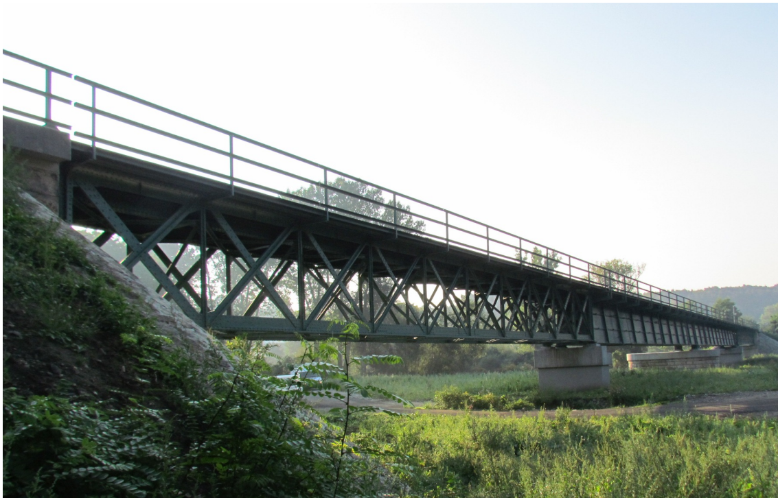
Figure 4.1: Bridge B1 – plate girder bridge with rail directly fixed to the top flange.
