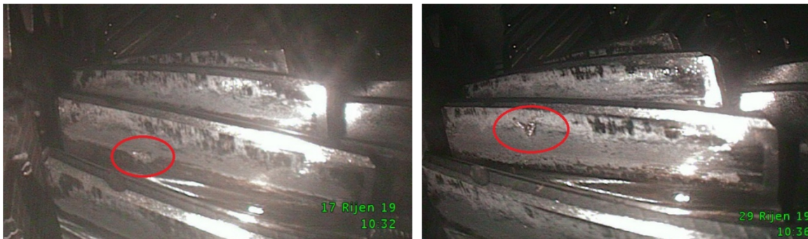
Figure 7-3: Pitting on PM HIP:ed gearwheel (3 rd speed pinion) – gearset 1 - after 115 hours (left), gearset 2 – after 100 hours (right)
