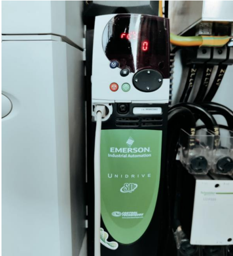
Figure 63 Emerson Control Unit
