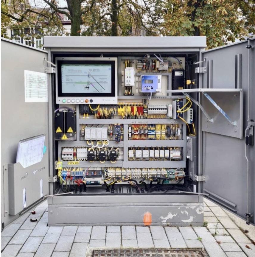
Figure 7: A deployed control cabinet [11]
