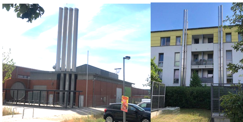
Figure 3.2.12 The Combined Heat and Power (CHP) Plants – standalone structure (left), included in apartment building basement (right) (source: Bardhyl Rama)
