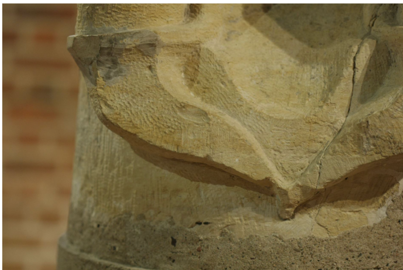
FIGURE 4. Old Town – Agnes Monastery, refectory, after 1234. Surface processing with toothed tools in a decorative grid (photo by M. Cihla, taken from [13]).
