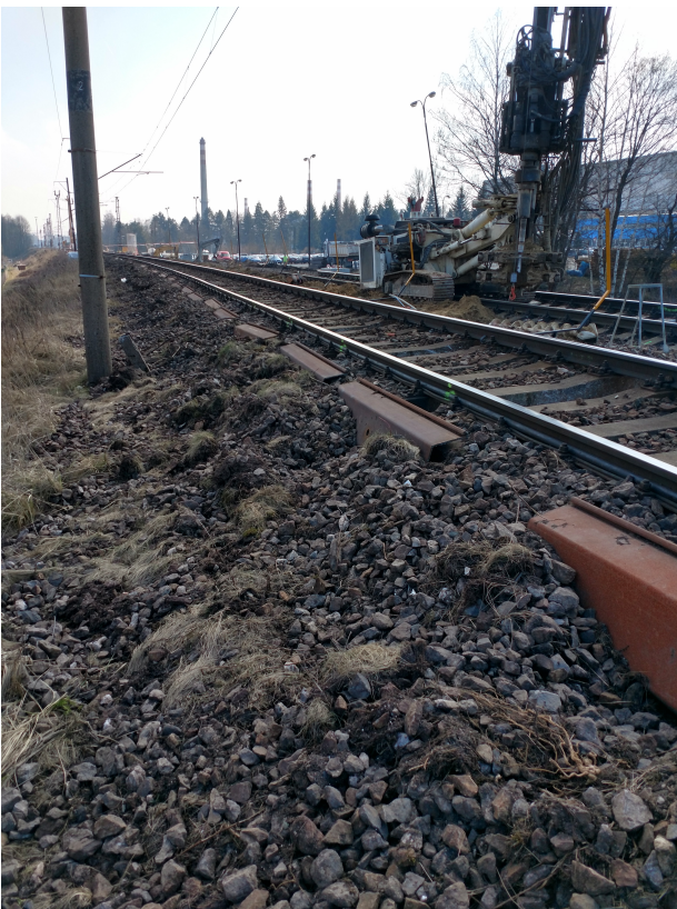
FIGURE 1. Condition of the railway before reconstruction: tilting of the traction line columns (top) and Temporary measures against disintegration of the track rail geometrical position (bottom).
