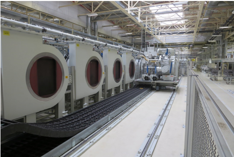
Figure 1.1: A steel hardening production line in Škoda Auto consisting of electrical vacuum furnaces [43].
