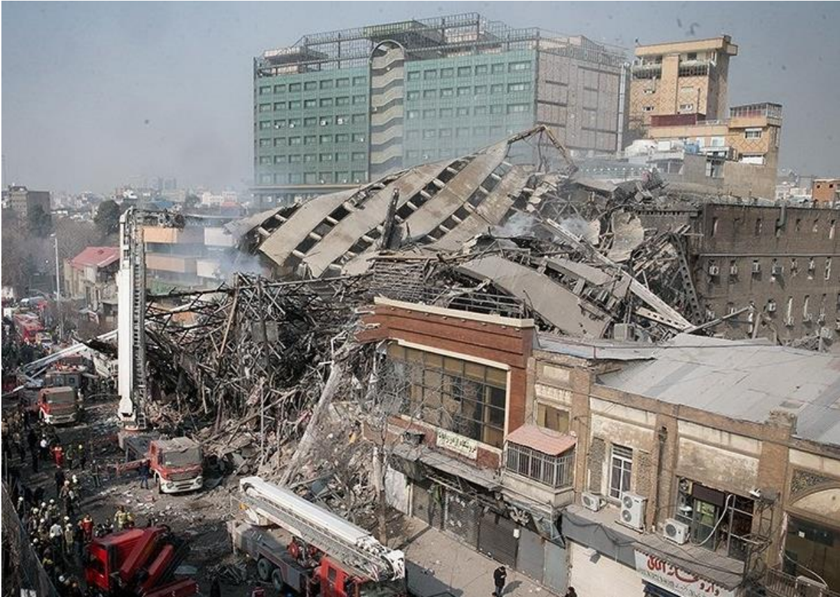
Fig. 1-7. Fire-induced collapse of Plasco building, Tehran 2017 [12].
