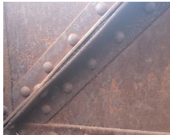
Fig. 4 Appearance of crevice corrosion
