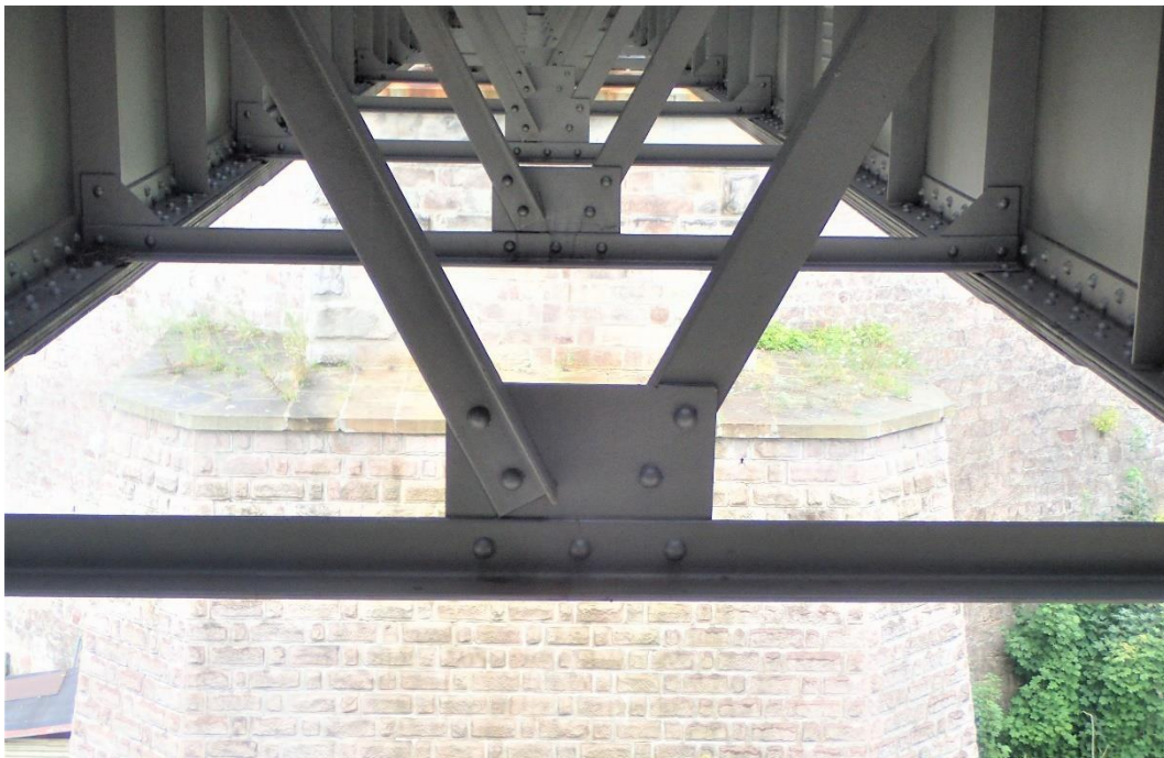
Fig. 40 Eccentric connection of vertical bracing members (steel riveted railway bridge in Trutnov).
