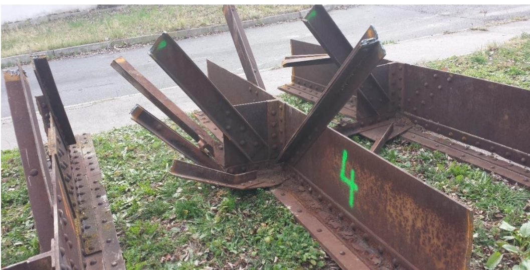
Fig. 28 Part 4 removed from the left-hand girder of the bridge structure
