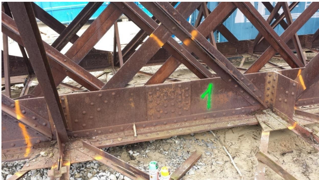
Fig. 25 Part 1 removed from the left-hand girder of the bridge structure
