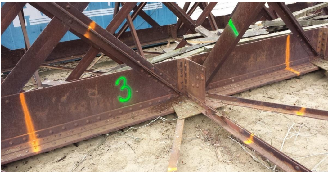
Fig. 27 Part 3 removed from the left-hand girder of the bridge structure
