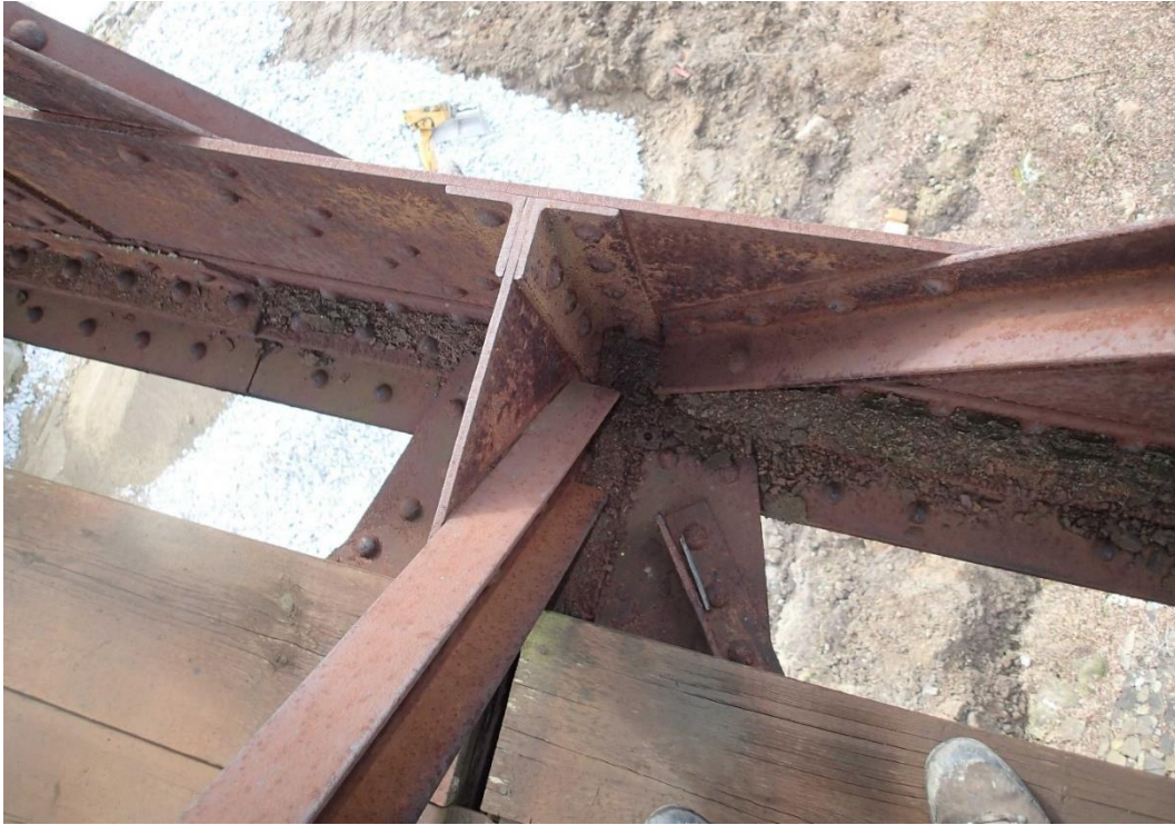
Fig. 41 Eccentric connection of diagonals to the bottom chord and eccentric connection of the vertical bracing member (steel riveted railway bridge in Holubov)
