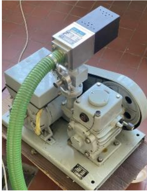
Figure 66: Vacuum pump used in CTU
