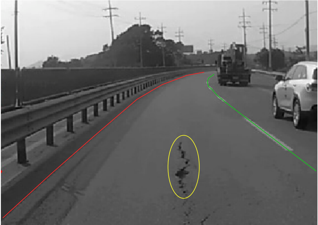
Figure 5.1: Road with a pothole adopted from [26]. In the figure, the detected limitations (environmental envelope) are presented. The red curve stands for the left road border. The green curve shows the right edge. Yellow color encircles boundary defined by a detected pothole. It is a circle from the top-view perspective and an ellipse from a driver's view.
