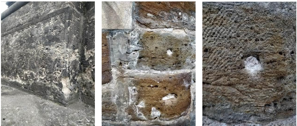
Figure 1: Example of stone weathering and salt damage near Charles Bridge, Prague Czech Republic
