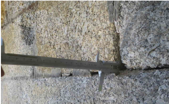
(a) : The mortar in the joints of the substructure is missing up to 200 mm deep.
