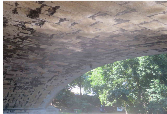
(b) : The salt leaching and deposits on the intrados of the vault (black because of SO_4^{2-} .)
