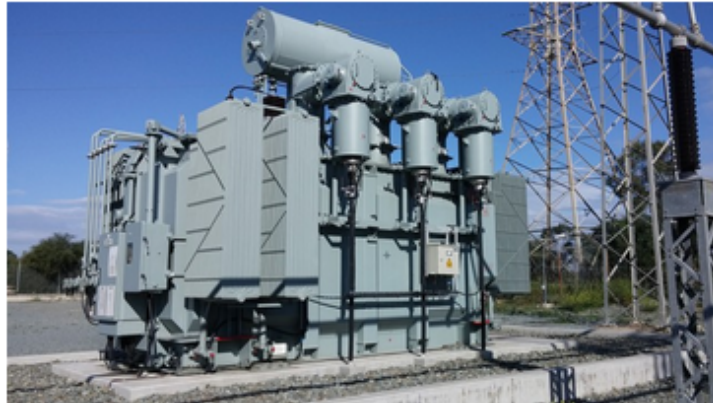
Figure 3.11: Variable Shunt Reactor [7]
