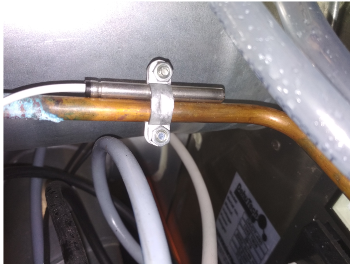
Figure 8: Improper installation of the temperature sensor at the refrigerant line
